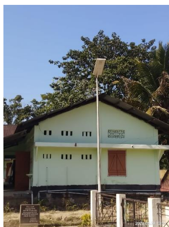
Fig. 5 Solar Street lights installed in the college campus
